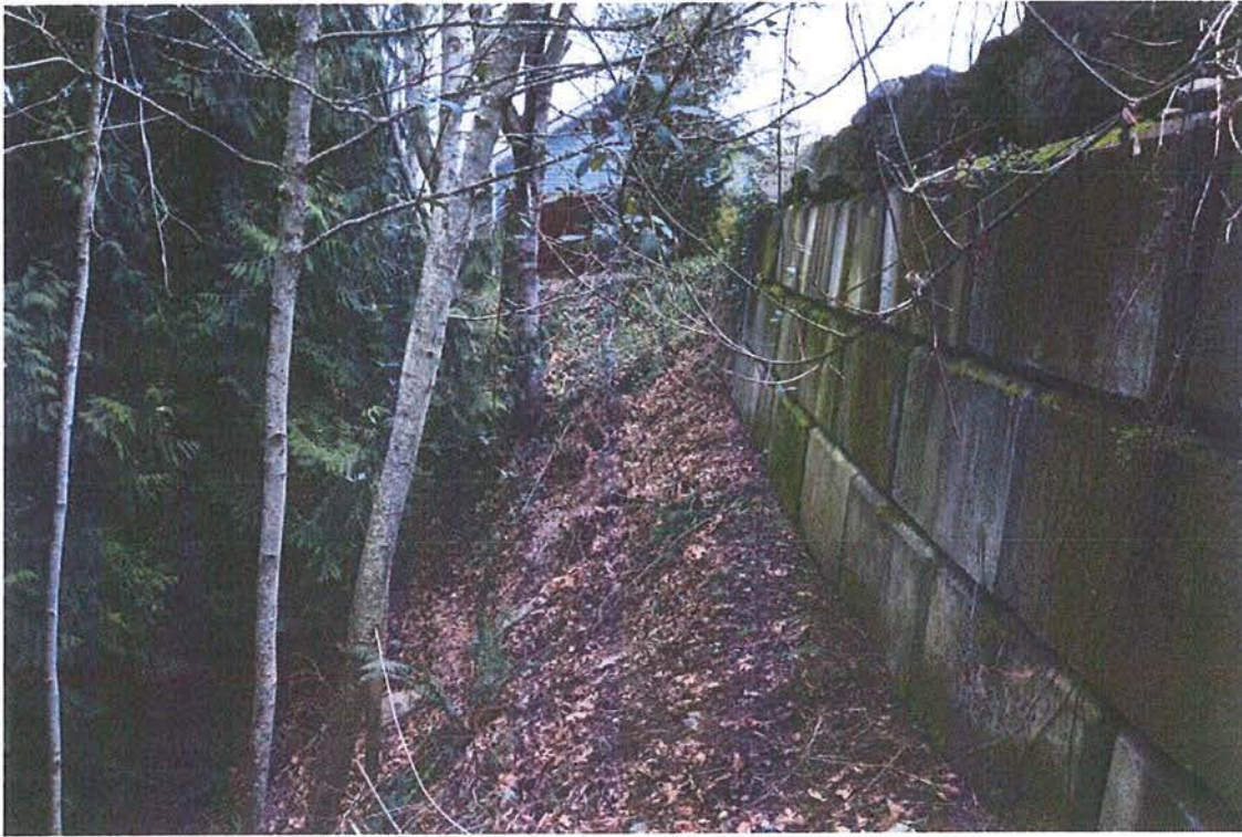
Figure 7: Retaining wall for adjacent land development along the 'top of bank' of Darough Creek.
